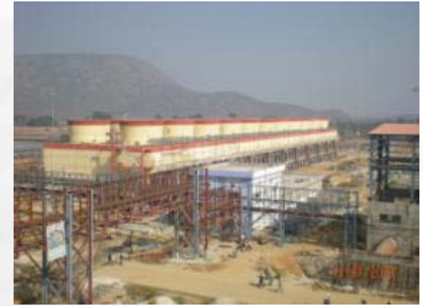
Induced Draft Cooling Tower
