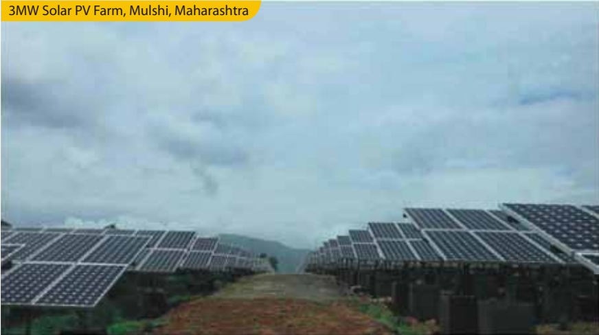
3MW Solar PV Farm, Mulshi, Maharashtra
