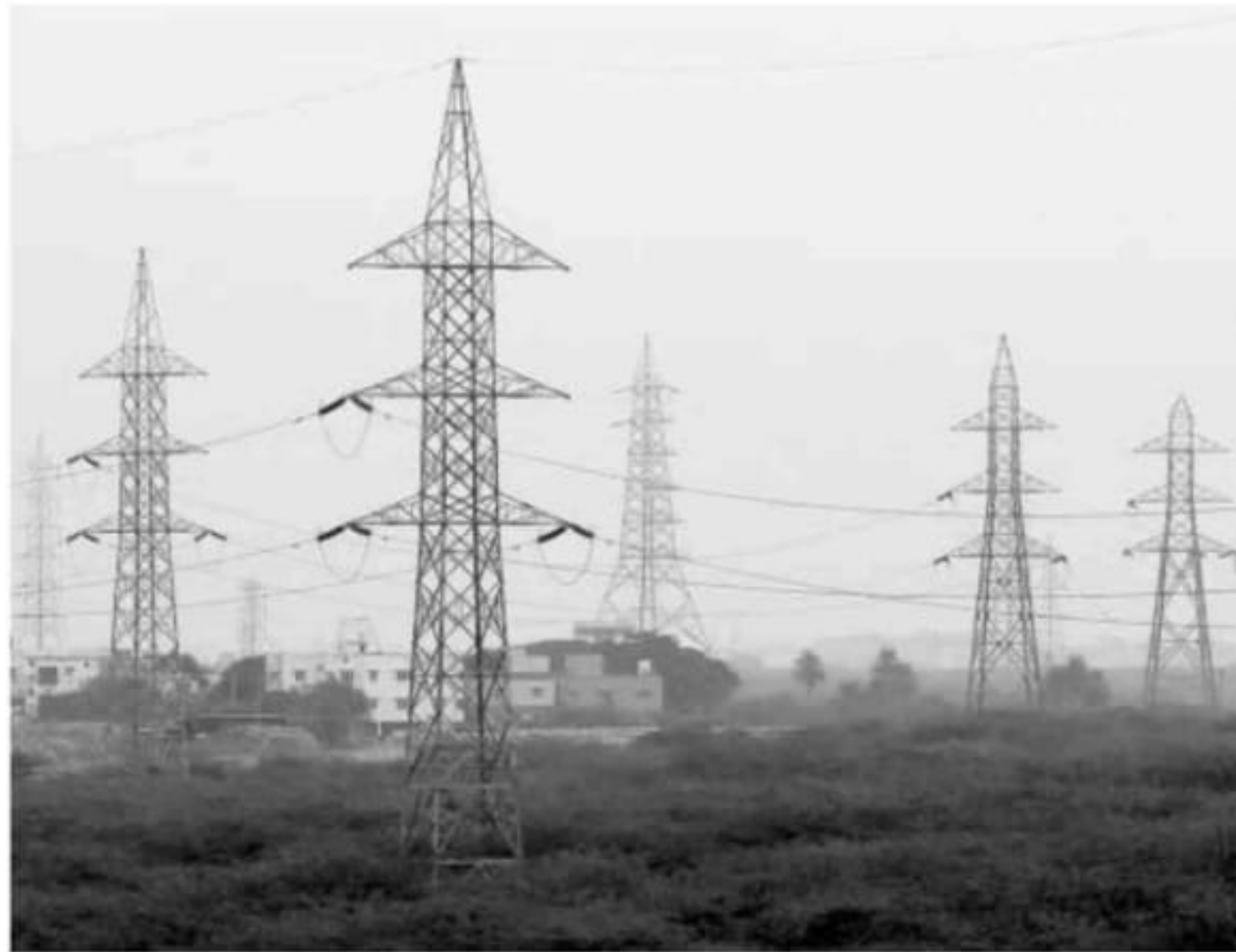
Discoms can improve reliability with better maintenance and advanced technologies
