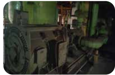
Heater drain pump with motor and pipes
