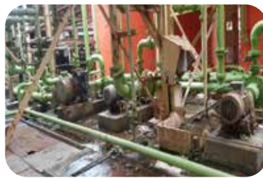
Boiler Pump for Storage Tank
