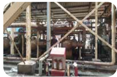
Load Carrying Oil and Stainer
