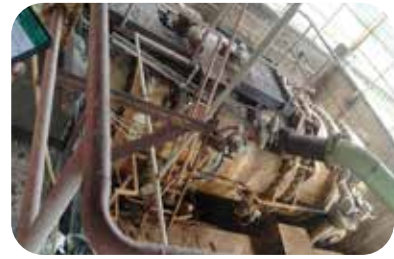
Inlet Condenser, Debris Filter
