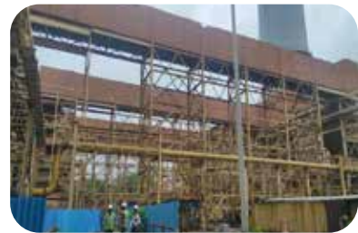
Flue Gas Duct
