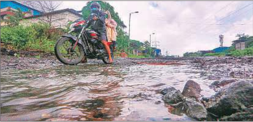
DIFFICULT JOURNEY: Commuters face a hard time as potholes have rendered Mahape MIDC Road in Navi Mumbai prone to accidents. Narendra Vaskar
